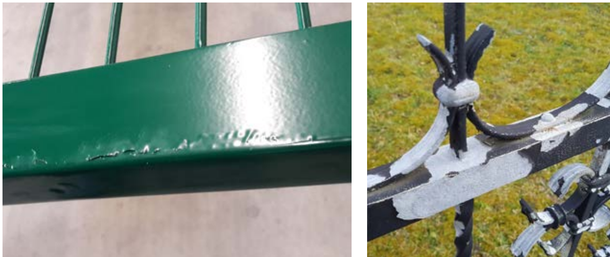
Figure 10: Zinc delamination after coating
