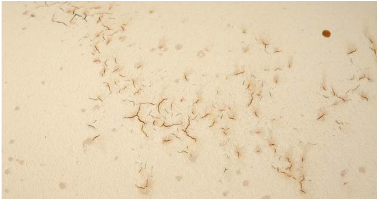
Figure 9: corrosion on substrate
