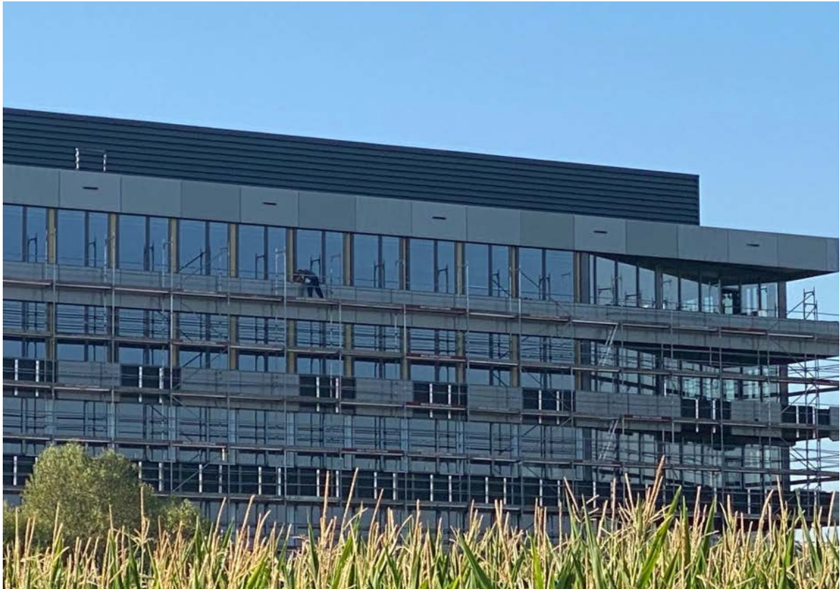
Figure 3 Colour deviation on a facade
