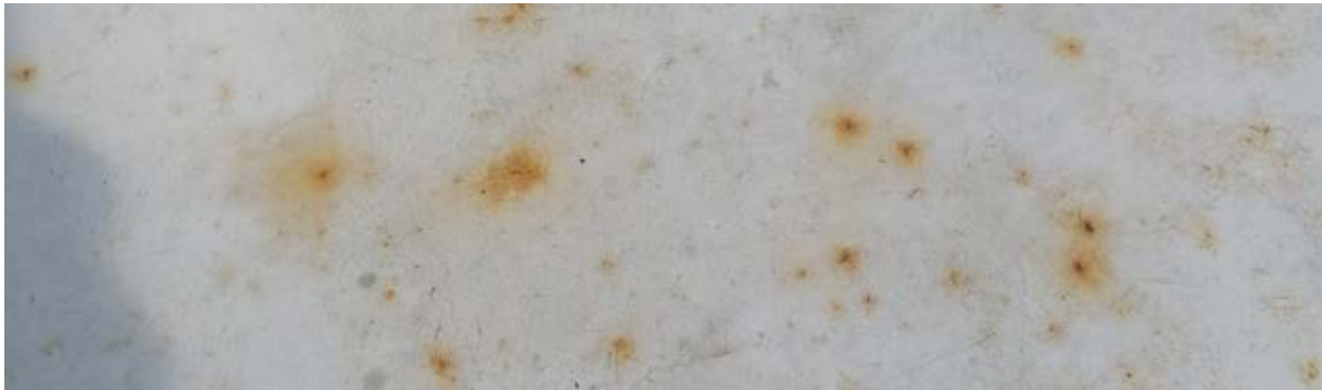
Figure 30: Corrosion damage due to insufficient coating thickness
