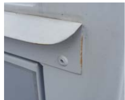
Figure 14: Damage caused by insufficient layer thickness at the edge
