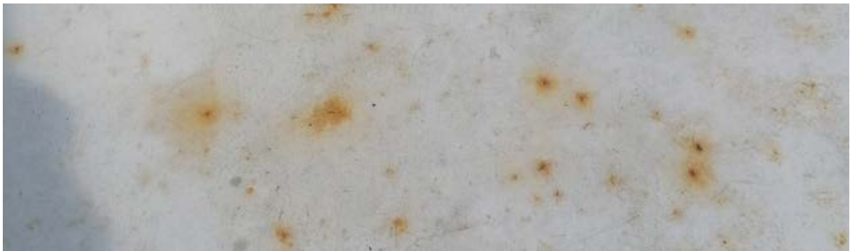
Figure 30: Corrosion damage due to insufficient coating thickness
