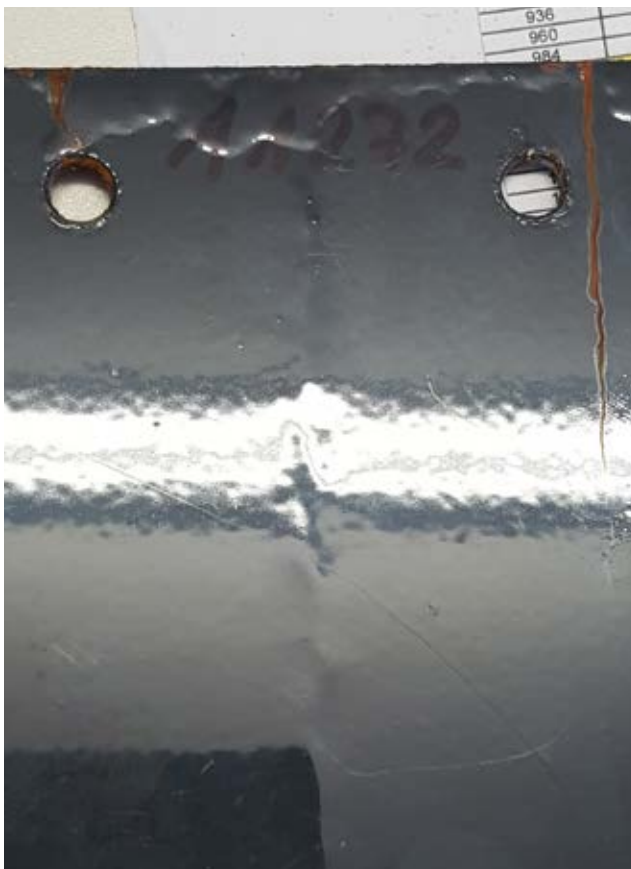
Figure 17: Corrosion problems at the edge area due to unprepared edges.
