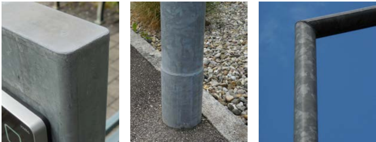
Figure 4: Examples for closed hollow components left: Metal post; middle and right: Detail shots of weld seams on a street lamp
