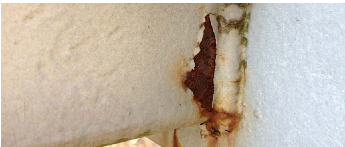
Figure 13: Coating damage on a weld seam that has not been properly cleaned.
