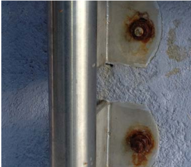
Figure 3: Example for contact corrosion: stainless steel handrail, galvanized screwing
